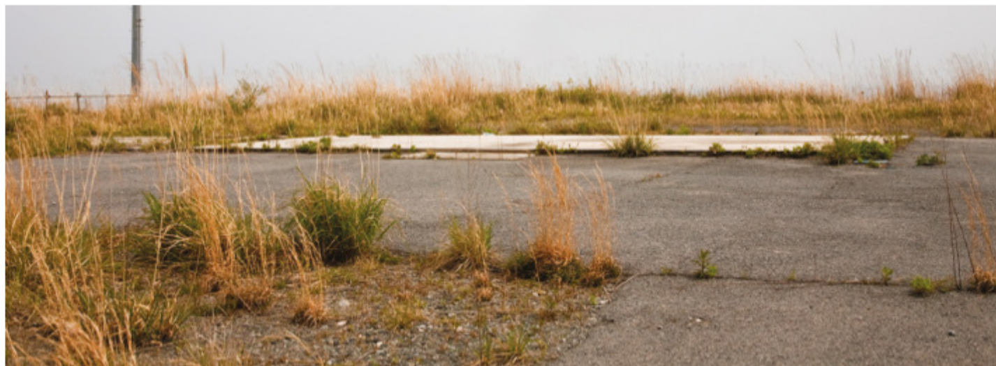
FIGURE 1.4.2 The grass closer to the concrete and in between the cracks in the concrete is green.
